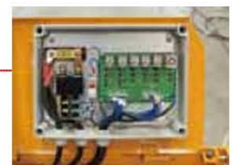
▶ Electric Control System
